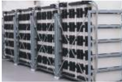
Energy Storage System
