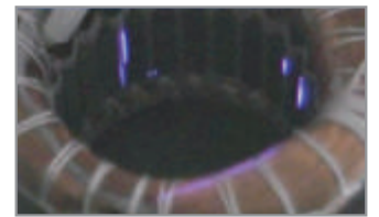
Figure 8 : Corona discharge in motor
